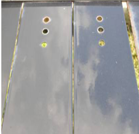
Figure 10 - Cracked and uncracked coatings specimens after exposure in south Florida.
