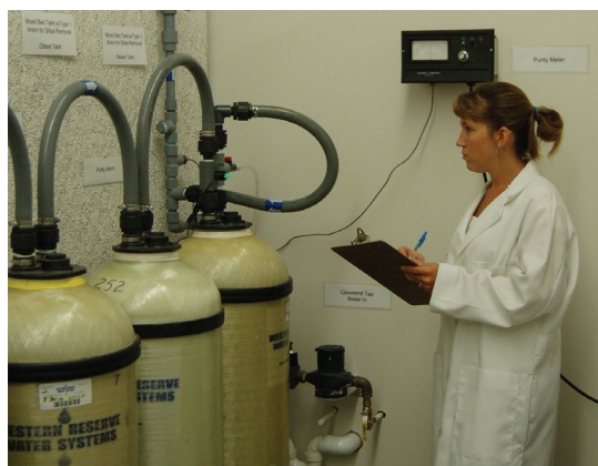
Large water purification system.
