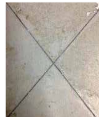
Paint applied to bare aluminum surface has completely delaminated
