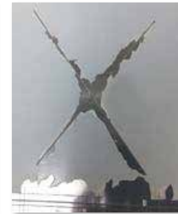
Aluminum panel made from alloy Y shows poor adhesion & significant delamination of paint from the surface
